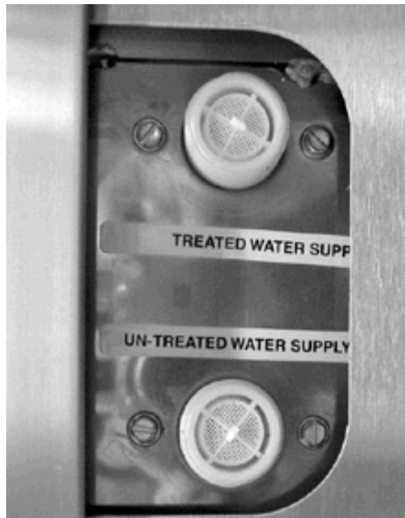
Standard water connections for steam generator and drain spray condenser.
