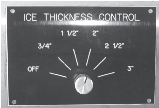
Ice Water Thickness Control Panel
